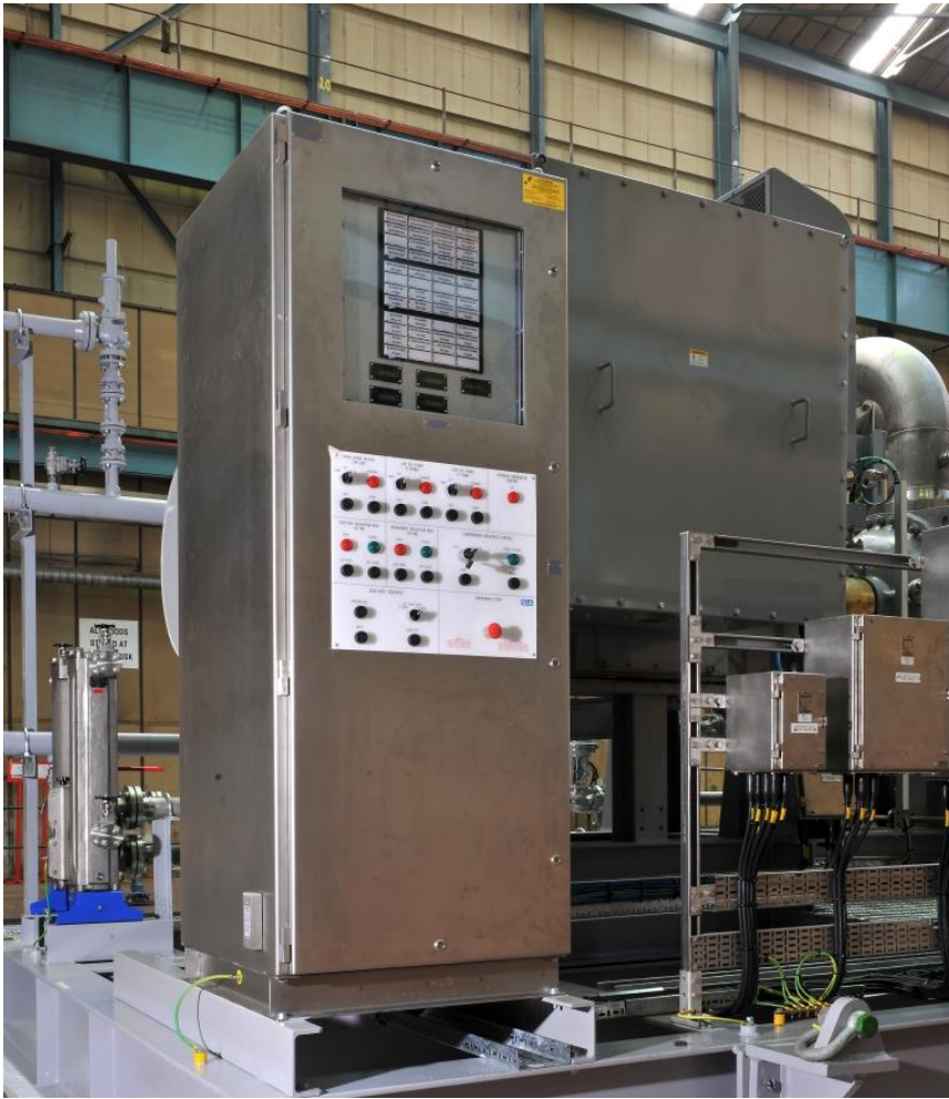
Figure 3: Showing the IEC 60079-2 Ex p pressurised local control panel with maintenance functions
