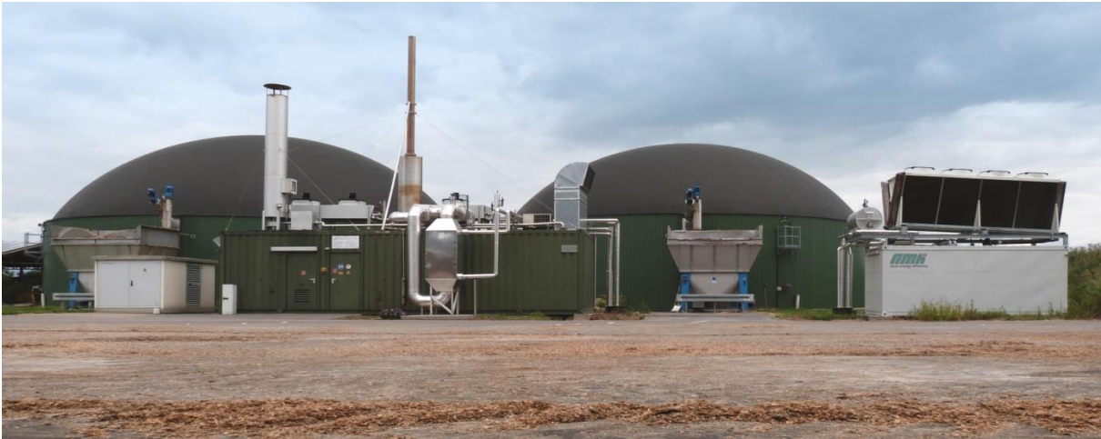
Fig. 3: Biogas plant in Pomerania (Northeast Germany) with a 500 kWe gas engine with an exhaust gas heat exchanger and an integrated IC60 ORC unit with an air cooled condenser.
